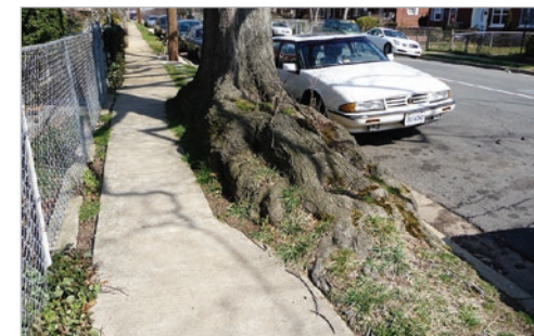
Constricted roots will find various places to grow including under paved infrastructure. Photo: VDOF
