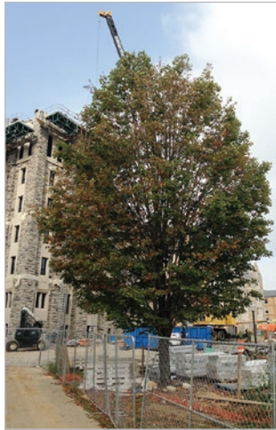
Construction activities compact the critical root zone. Photo: Eric Wiseman, Virginia Tech
