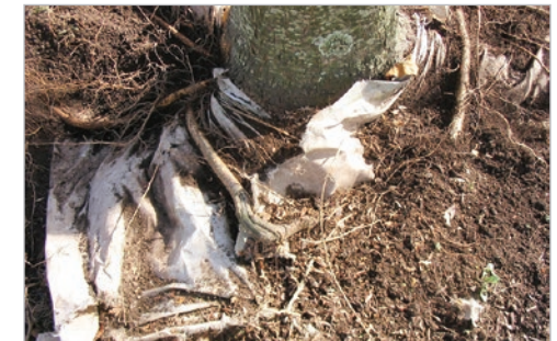
Root barrier struggles to stretch as the tree grows with age. Photo: Joe Murray, Treebio.com, Bugwood.org
